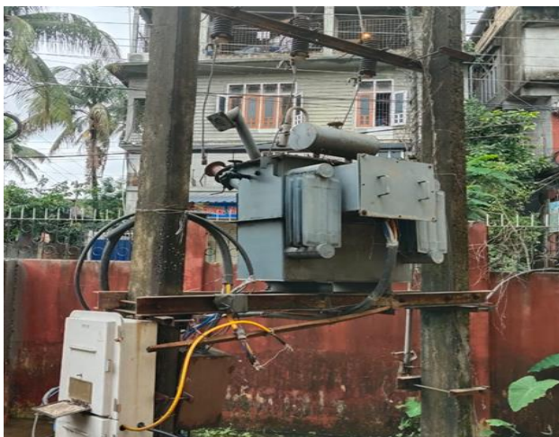
Installed transformer (100 kVA) inside the college campus
