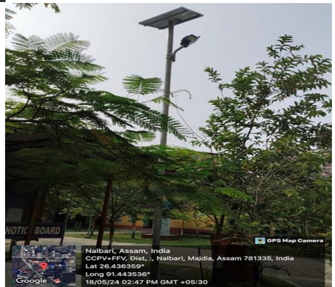
Solar street light in the college campus
