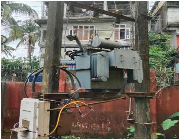
Installed transformer (100 kVA) inside the college campus
