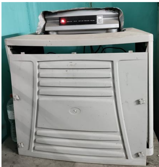
Inverter with battery as a source of energy storage
