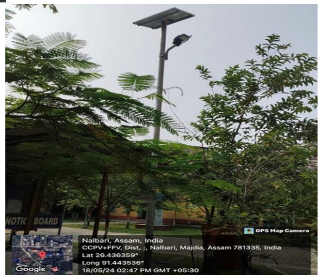
Solar street light in the college campus
