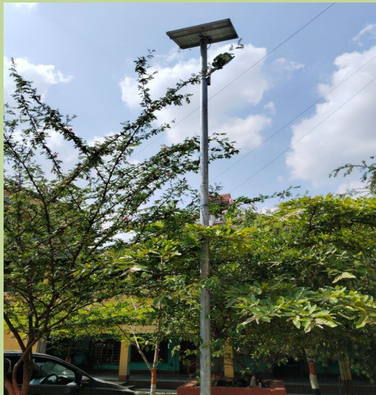
Installation of solar-powered street lights on campus as part of the Green Energy Mission, promoting awareness of renewable energy for a sustainable future
